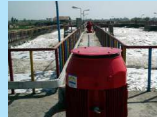
WASTE WATER TREATMENT 500 M 3 /HOUR
